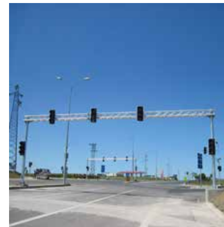
TAG SIGNAL POLE
